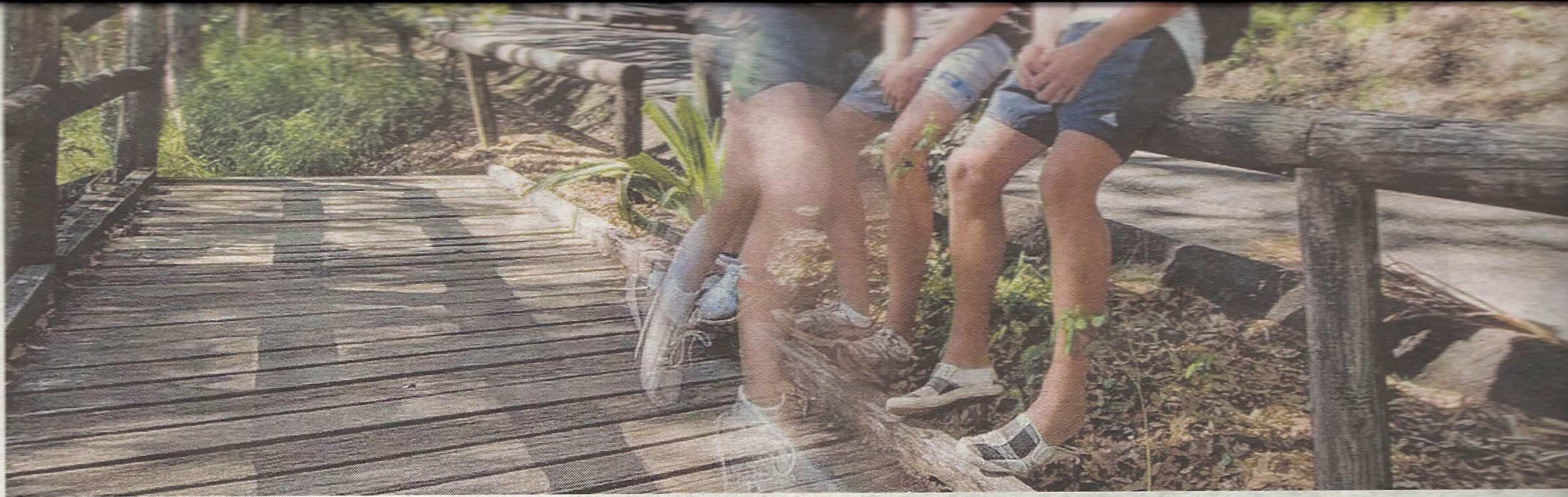
LEVEL PEGGING: Tourists Jacko Nelson, 14, (left) and Chris Spratt, 14, on the leaning boardwalk alongside Park Rd at Noosa. Picture: John
